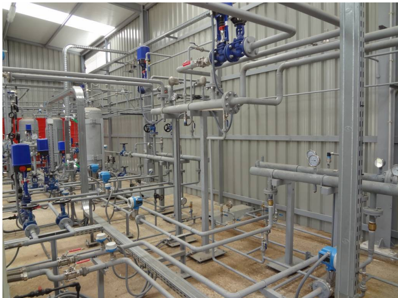
Figure 2.19: Hydraulic installation (extracted from D5.2)
